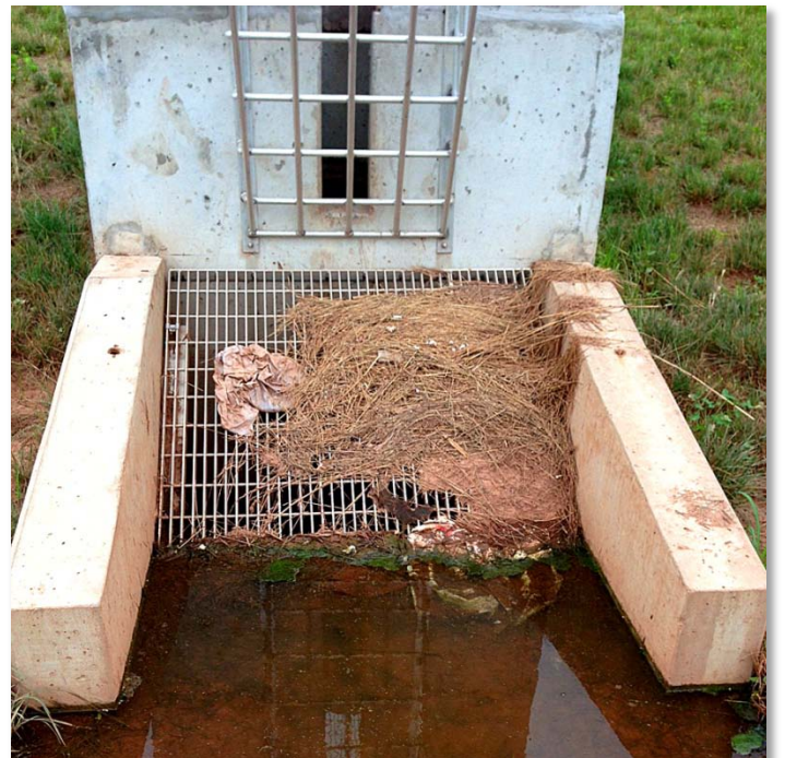
Small openings in trash racks clog more easily. The smaller the openings, the more frequent inspections and maintenance are required.
