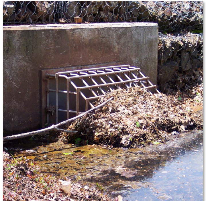
Clogged trash racks can block water flow into the Outlet Control Structure causing flooding and damage to the system.
